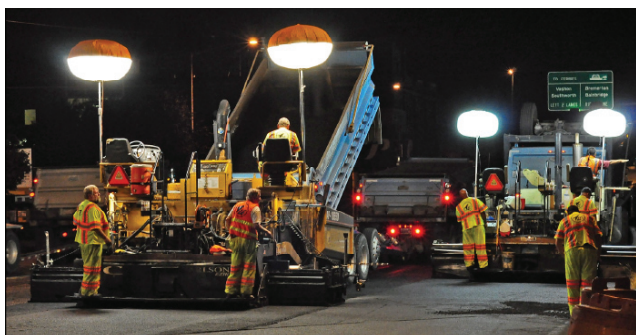
WMA Paving on 4th Ave S. (note lack of fumes) Photo Credit: City of Seattle
